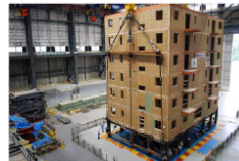
The capstone test structure is moved onto the E-Defense shake table in Japan on June 22, 2009. Photo courtesy of John van de Lindt, Colorado State University.
