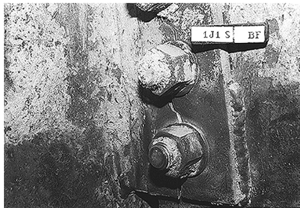
Figure 1-5 Vertical Fracture through Beam Shear Plate Connection
