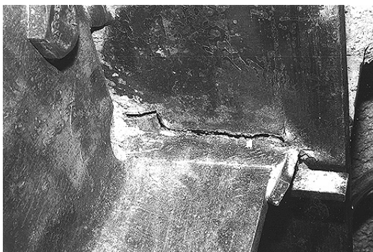
a. Fracture at Fused Zone
