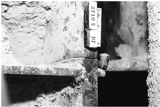
a. Fractures through Column Flange
