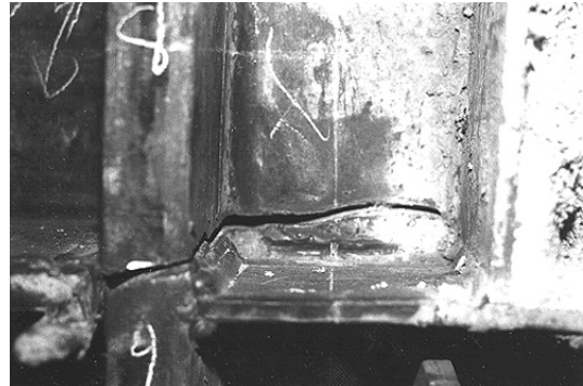
b. Fracture Progresses into Column Web
