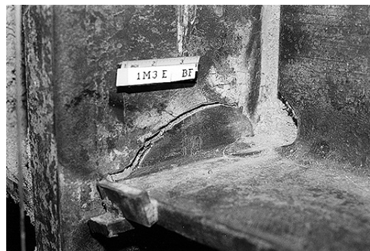
b. Column Flange "Divot" Fracture
