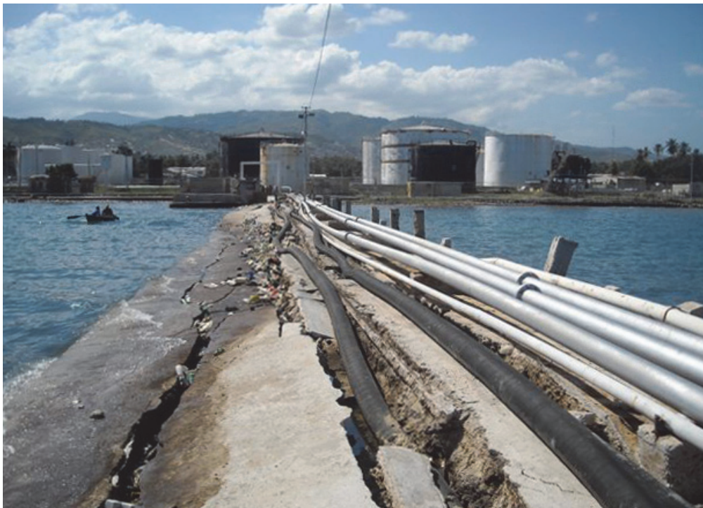
Figure 2-6 Embankment-supported petroleum pipelines, Port de Port-au-Prince, impacted by the 2010 Haiti earthquake (Source: Scott Chodkiewicz, U.S. Army Corps of Engineers).
