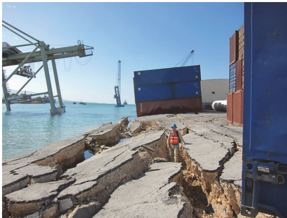
Figure 2-3 Fissures caused by lateral spreading, Port de Port-au-Prince, during the 2010 Haiti earthquake (S. Baldrige photograph).
