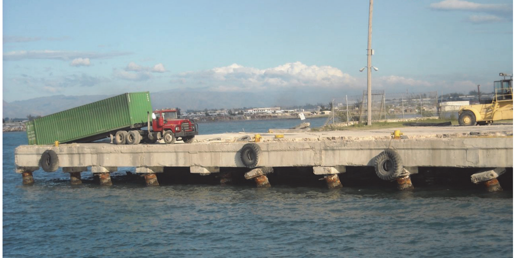
Figure 2-7 Remaining portion of pile-supported pier at the Varreux terminal, Port de Port-au-Prince, following the 2010 Haiti earthquake (Source: Scott Chodkiewicz, U.S. Army Corps of Engineers).
