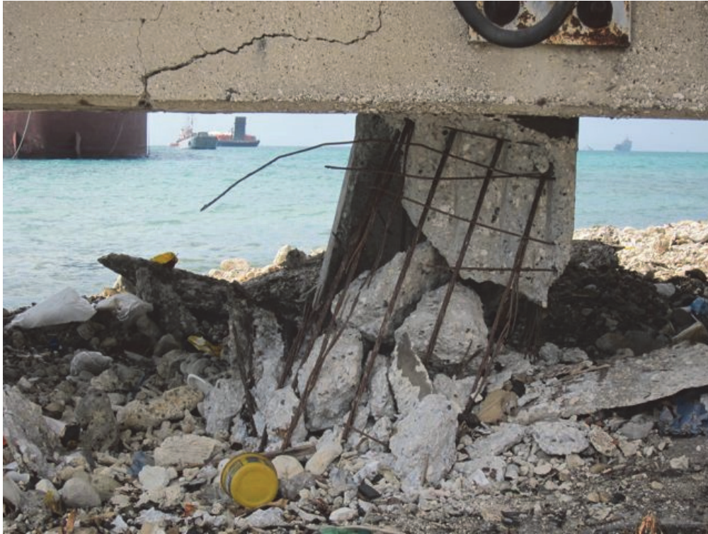
Figure 2-5 Extensive damage to the landward row of piles, Port de Port-au-Prince, caused by the 2010 Haiti earthquake.
